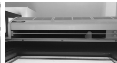
Air curtain in supermarket
