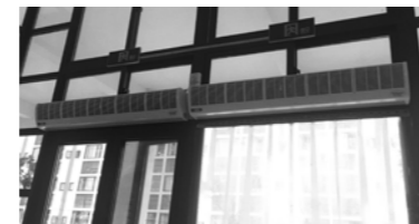
Air curtain in dining hall
